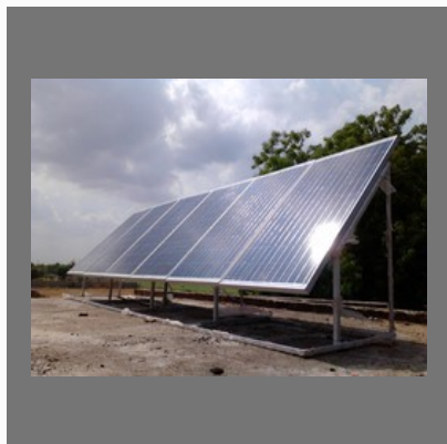
Solar Rooftop 10kw
