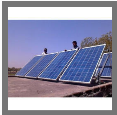
Solar Roof Top Power Plant
