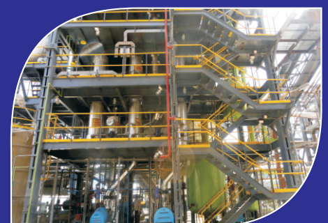
Multi Effect Evaporator Plant (MEE)
