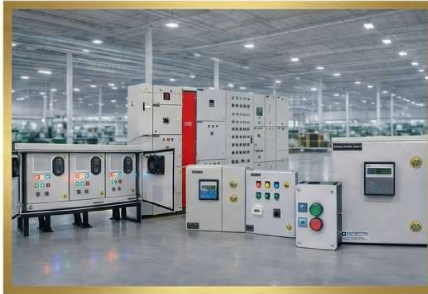
Power Factor & Backup: APFC, AMF, and DG Synchronisation Panels.
