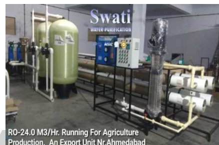
RO-24000 LPH (24 M3/Hr)
