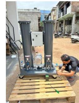
Fuel Treatment Plant
