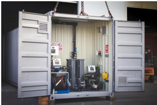
containerised fuel station with filtration
