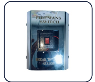
Emergency Alarm with Battery
