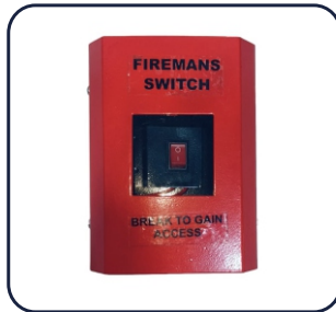
Fireman Switch (MS)
