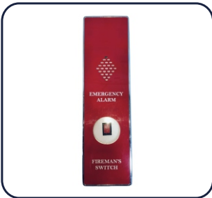
Emergency Alarm & Fireman Combo
