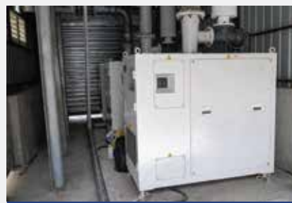
Banas Dairy WWTP Project
