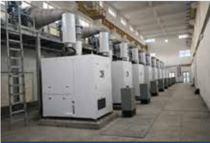
564 MLD Okhla WWTP Plant
