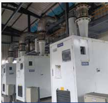
ETP Plant Huber Group
