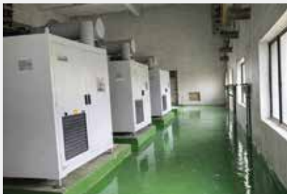
60 MGD Keshopur STP Plant
