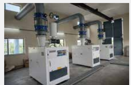
16 MLD Sayaji Garden Plant
