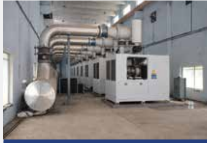
150 MLD K&C valley STP
