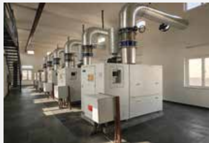
60 MLD Jaspur STP Plant
