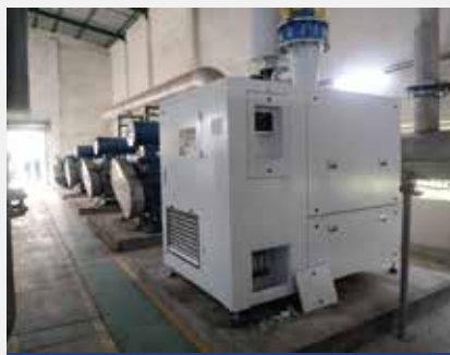
Budhni ETP Plant
