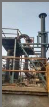
HDPE scrubbing system
