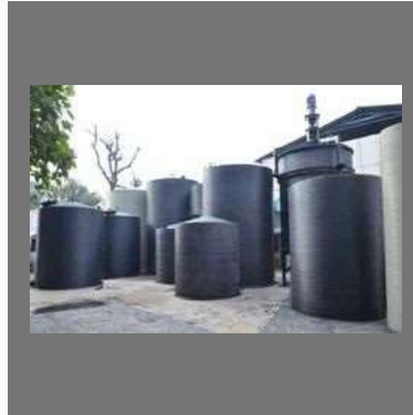
Spiral Vertical HDPE Storage Tanks
