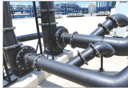
PP FRP Duct with Blower Assembly
