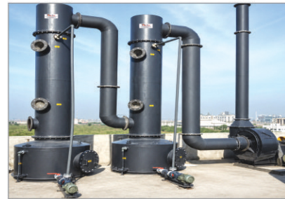
Ammonia Gas Scrubber
