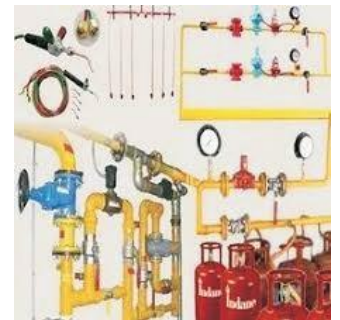
LPG GAS PIPELINE
