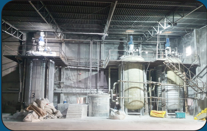
Liquid Sodium Silicate Plant
