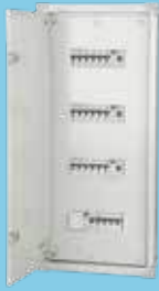
VERTICAL PER PHASE ISOLATION DOUBLE DOOR DB
