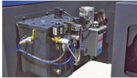
Mist Cooling System
