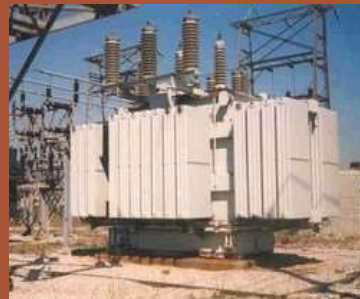
Electrical Power Transformer
