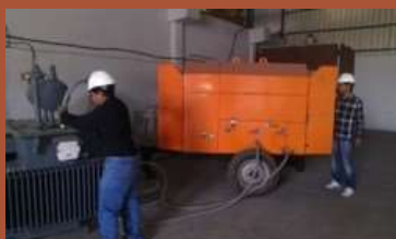
Online Transformer Oil Filtration
