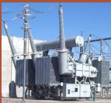
Step Up Transformer
