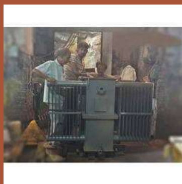
Transformer Leakage Attended Services
