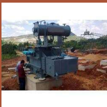
Transformer AMC Service
