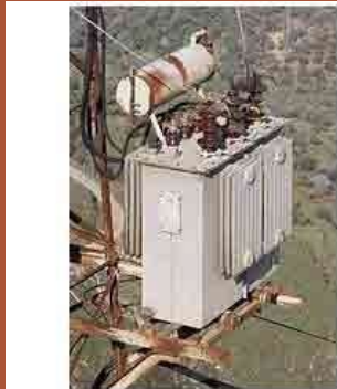
Constant Voltage Transformer
