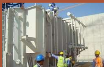
Onsite Transformer Maintenance Services
