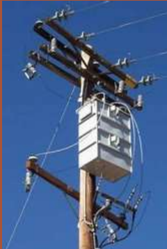
Step Down Transformer
