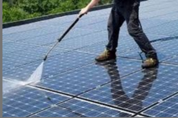
Solar Panel Cleaning System
