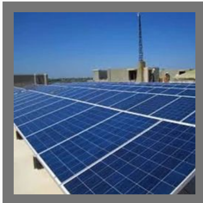
Off Grid Solar Power Plant
