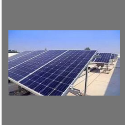
Solar Rooftops System
