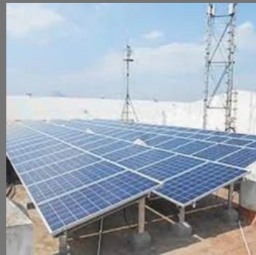
Off Grid Solar System
