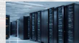
Data Center Cooling
