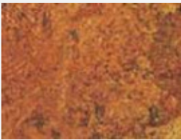
Mill scale on steel surface has rusted away, but with slight pitting visible under normal vision.
