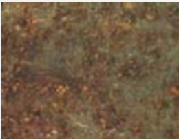
Steel surface has begun to rust and mill scale has begun to flake.
