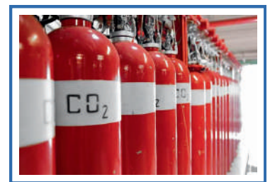
Co2 Fire Suppression/Flooding System
