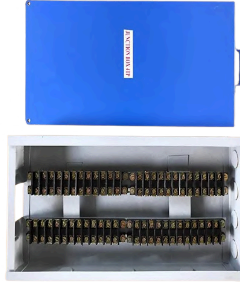
Inspection Box ( 4TP) AI-03
