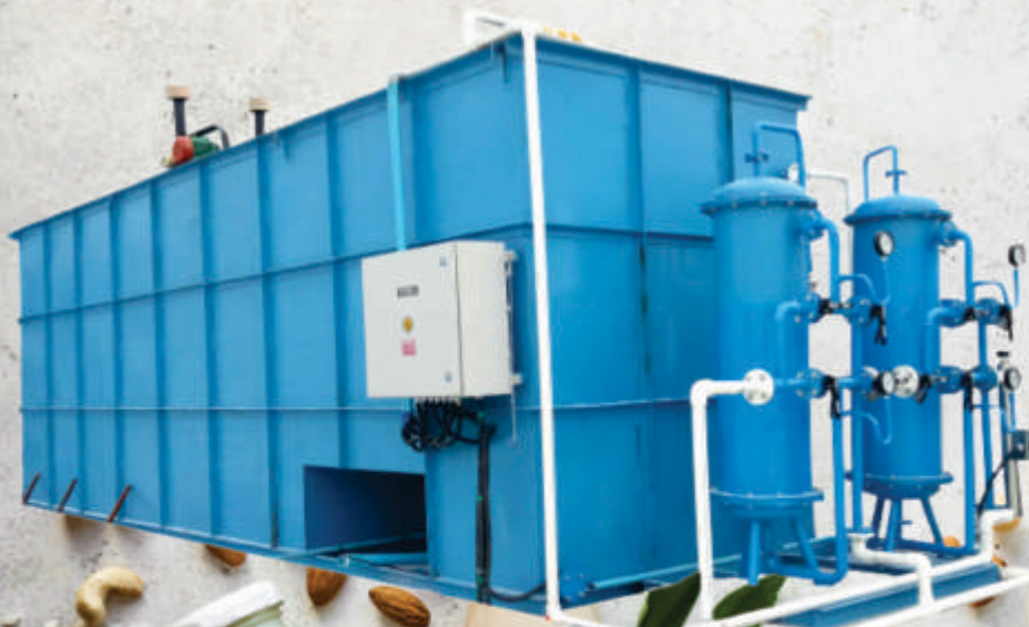
EFFULENT TREATMENT PLANT
