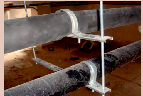
G.I. Piping Supports
