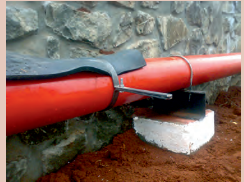
M.S. Piping Supports
