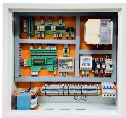
Elevator Geared Controller
