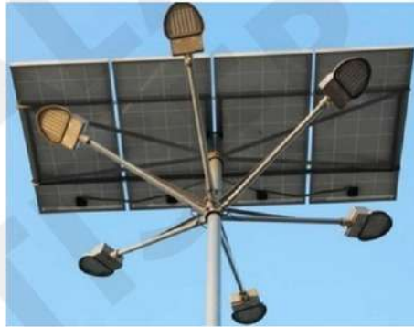
Solar High Mast Light
