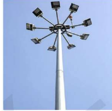
High Mast Light
