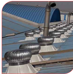
Roof Top Air Ventilator
