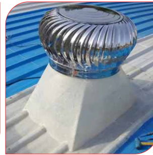
Turbine Air Ventilator
