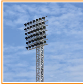
Highmast & Stadium Pole
