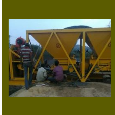
Mobile Hot Mix Plant
