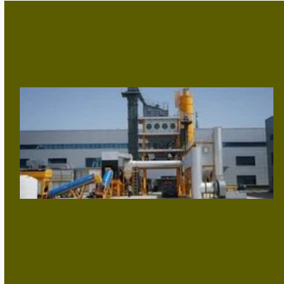
Asphalt Batch Mixing Plant
